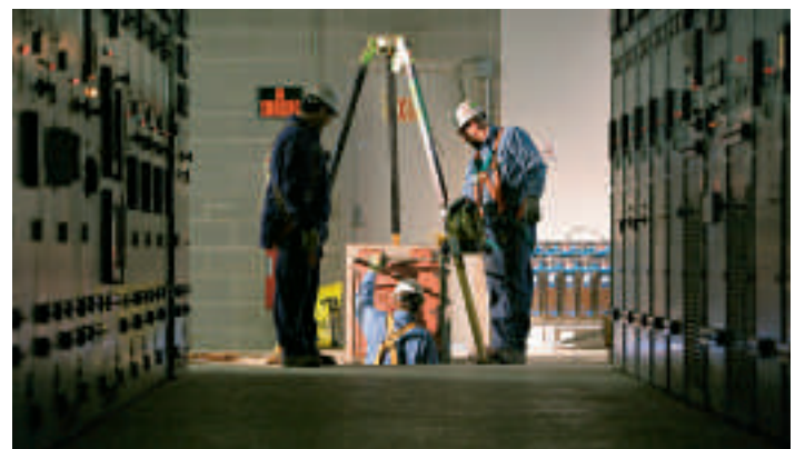
Descending into a substation with special equipment.
